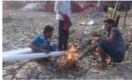
Figure 4 Burning of PVC pipe at bottom before installation
